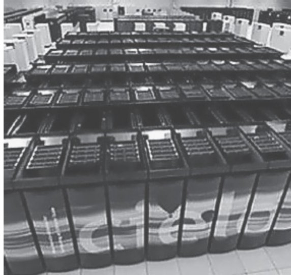
Cielo supercomputer at Los Alamos *15
